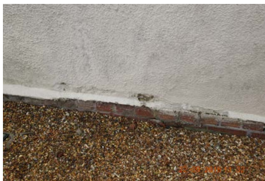
Photo 10 – Damage to low level render on rear north western elevation
