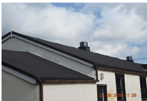
Photo 6 – Rudimentary arrangement of flashing between roof over store and main hall. Undulations in ridge of main roof also clearly evident in this photo.
