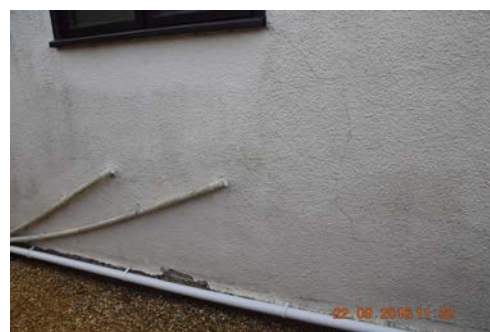
Photo 9 – Typical fine cracking below window in rear north western elevation
