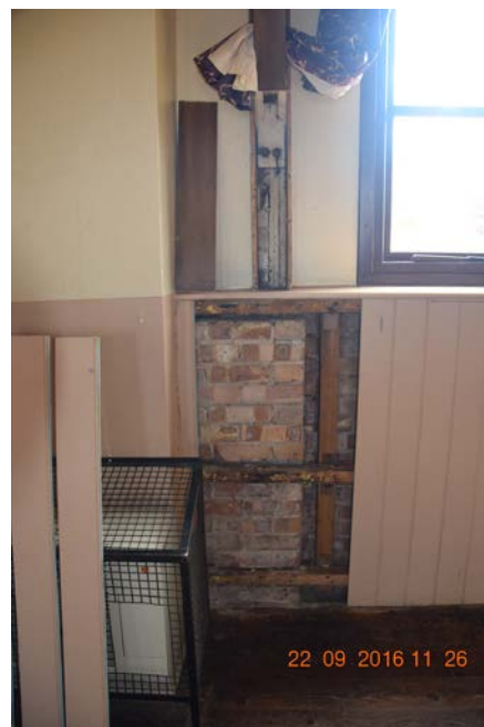
Photo 18 – Column and low level wall exposed on front elevation adjacent to the redundant fireplace
