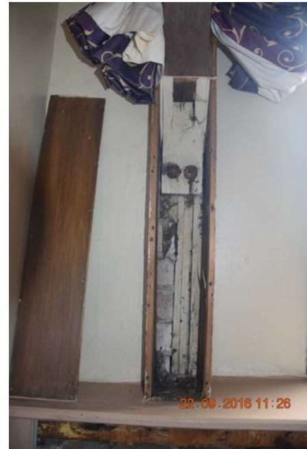
Photo 20 – Timber column above low level wall indicating multiple timber stud and steel bolts but no reinforcing steel column
