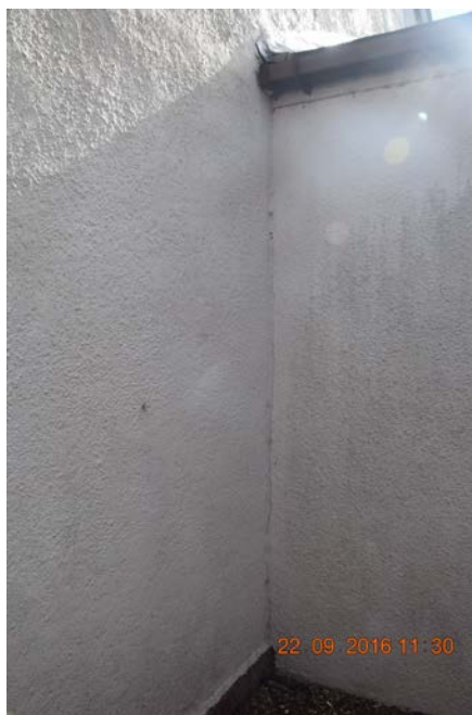
Photo 7 – Vertical joint at junction of store extension with main hall
