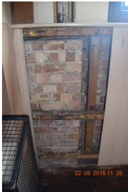
Photo 19 – Low level wall adjacent to redundant fireplace with horizontal timbers containing some rot
