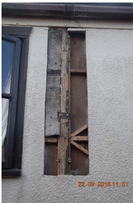
Photo 12 – Section of external render removed at location of internal truss and post at position indicated on drawing 167625 / 01
