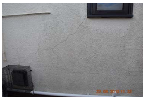
Photo 8 – Fine cracking in rear north western elevation
